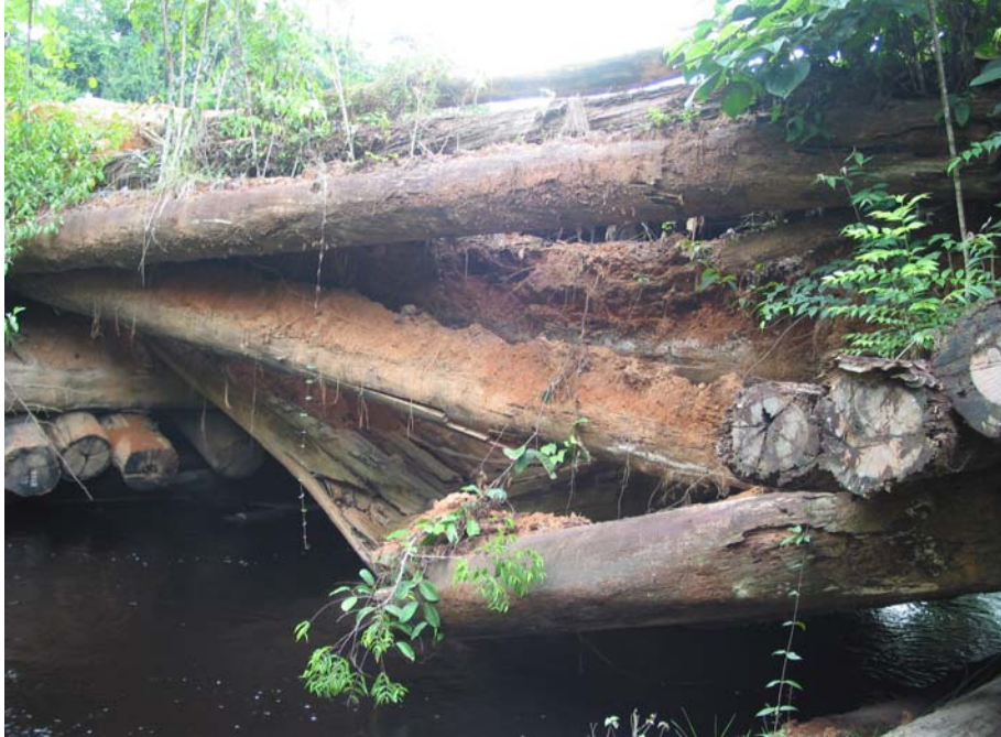
Figure 4: Photograph showing degradation of a bridge
