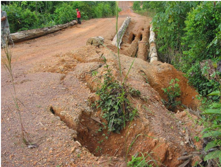
Figure 3: Photograph showing severe erosion near a bridge
